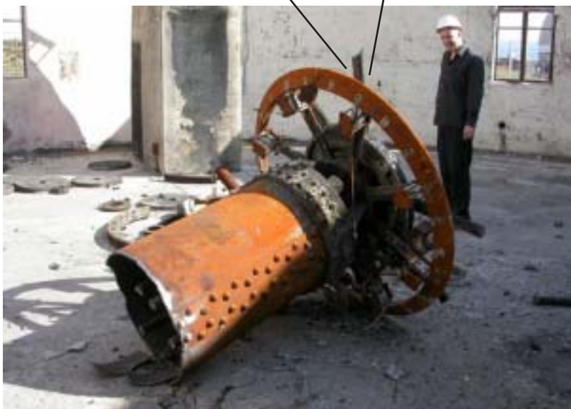
The original concept (top left) and damage to the RA wheel and drive gear that only became apparent on removal and which render this design impractical
